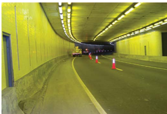
Figure 31. Tunnel lighting and white tunnel walls in Washington, DC (Source: FHWA 2005).
