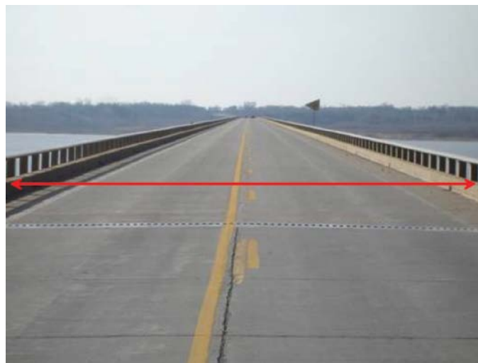
Figure 30. Bridge with narrow lateral clearance (Source: Albin et al. 2016).
