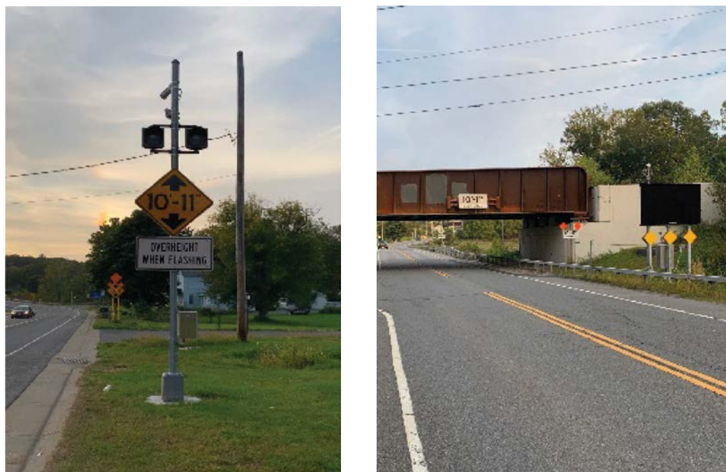
Figure 37. Components of an early warning detection system installed in Glenville, NY (Source: VHB).
